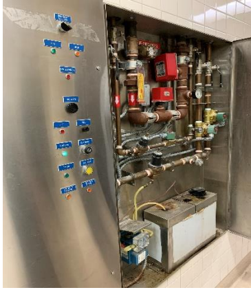
Kitchen Wash Control Panel Condition
