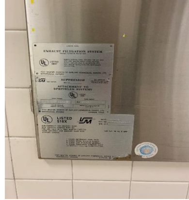
Kitchen Wash Control Panel Condition
