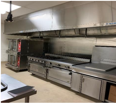
Kitchen Equipment Condition
