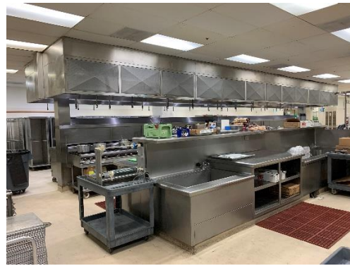
Kitchen Equipment Condition
