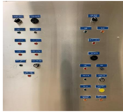
Kitchen Wash Control Panel Condition
