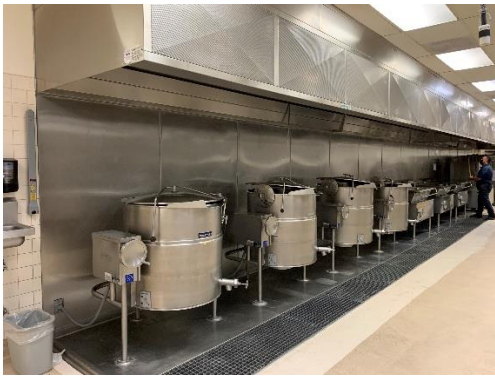
Kitchen Equipment Condition
