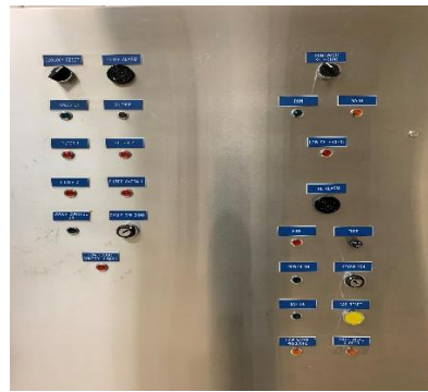
Kitchen Wash Control Panel Condition
