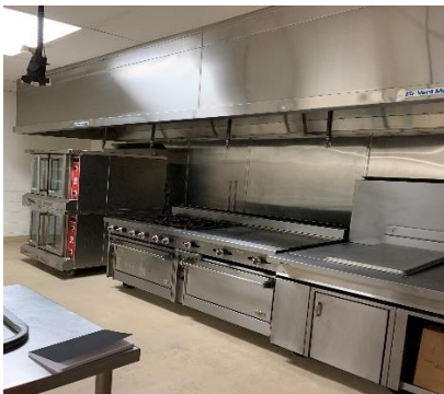
Kitchen Equipment Condition
