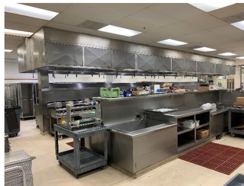
Kitchen Equipment Condition
