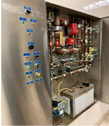
Kitchen Wash Control Panel Condition
