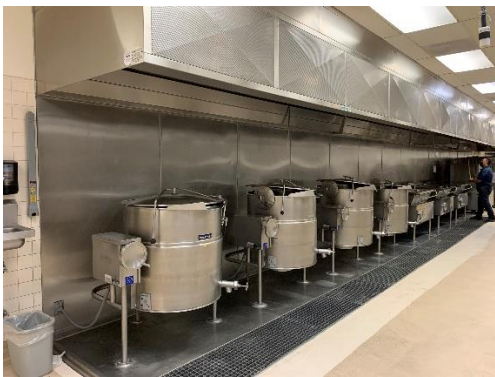
Kitchen Equipment Condition
