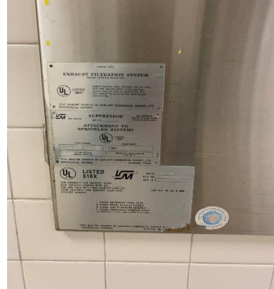
Kitchen Wash Control Panel Condition
