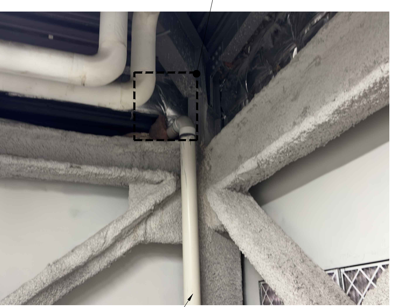
NOTES: 1. INSULATION REMOVED SHALL BE REINSTALLED AFTER PLUMBING WORK IS COMPLETE. AND DAMAGED INSULATION SHALL BE REPLACED IN MATCHING TYPE, AND THICKNESS. 2. REPLACE DAMAGED FIREPROOFING IN LIKE KIND. DRAIN LOCATIONS PHOTO REFERENCE 8 WP9.03 N.T.S. DO NOT SCALE PHOTO REFERENCES.
