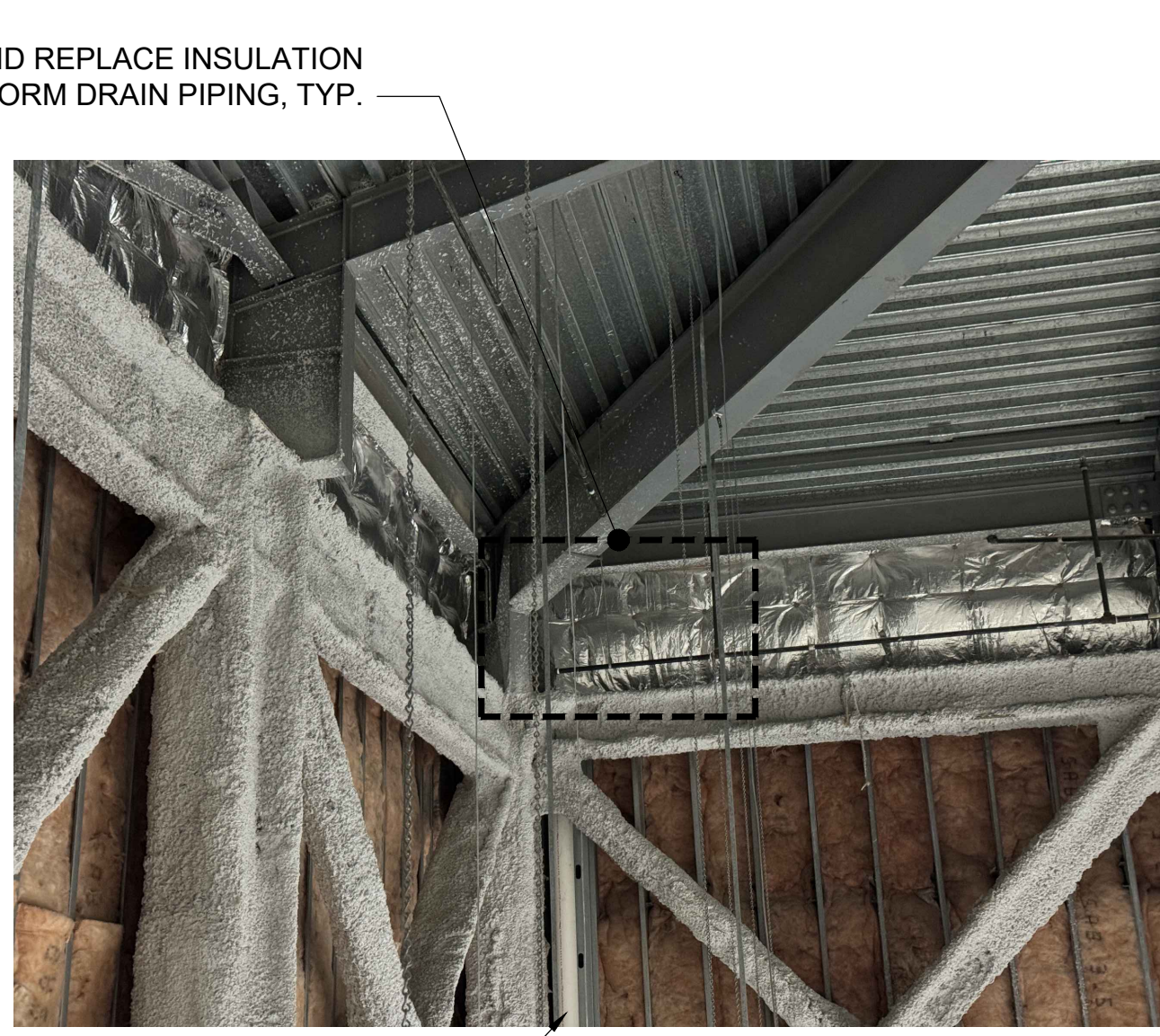
NOTES: 1. INSULATION REMOVED SHALL BE REINSTALLED AFTER PLUMBING WORK IS COMPLETE. AND DAMAGED INSULATION SHALL BE REPLACED IN MATCHING TYPE, AND THICKNESS. 2. REPLACE DAMAGED FIREPROOFING IN LIKE KIND. DRAIN LOCATIONS PHOTO REFERENCE 1 WP9.03 N.T.S. DO NOT SCALE PHOTO REFERENCES.
