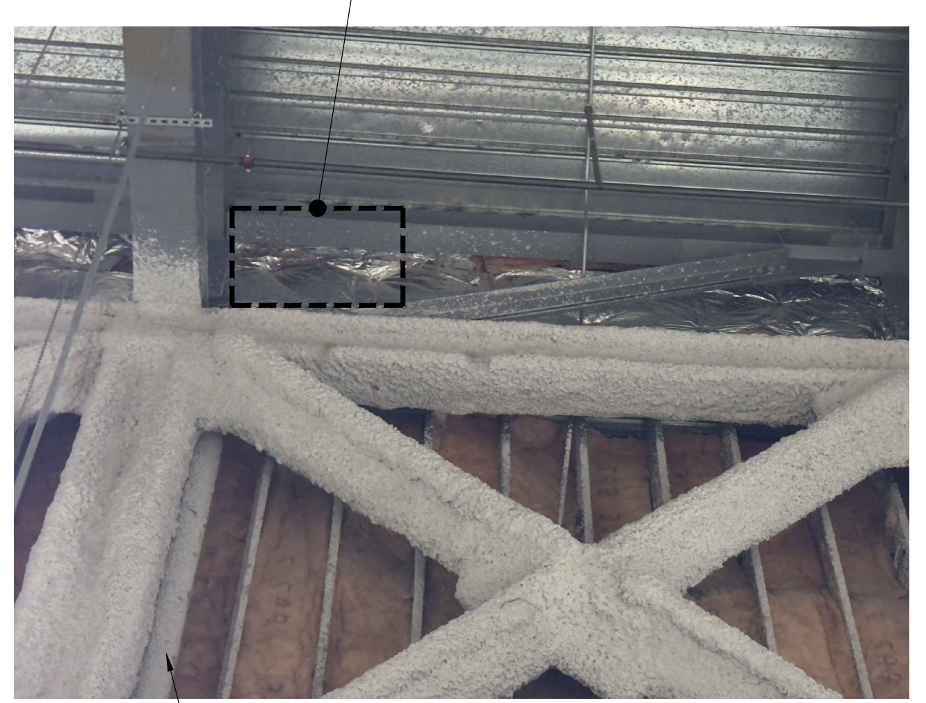
NOTES: 1. INSULATION REMOVED SHALL BE REINSTALLED AFTER PLUMBING WORK IS COMPLETE. AND DAMAGED INSULATION SHALL BE REPLACED IN MATCHING TYPE, AND THICKNESS. 2. REPLACE DAMAGED FIREPROOFING IN LIKE KIND. DRAIN LOCATIONS PHOTO REFERENCE 11 WP9.03 N.T.S. DO NOT SCALE PHOTO REFERENCES.
