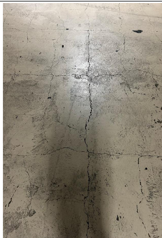
Various cracking throughout parking garage to be repaired/sealed prior to new floor sealing.
