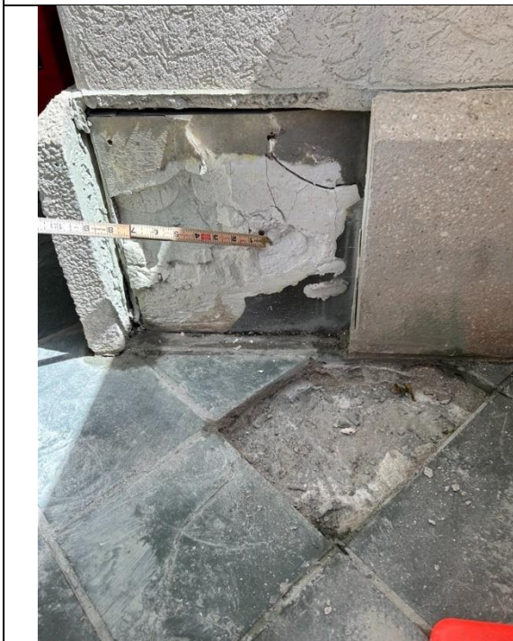
Stone Base – Damaged Substrate
